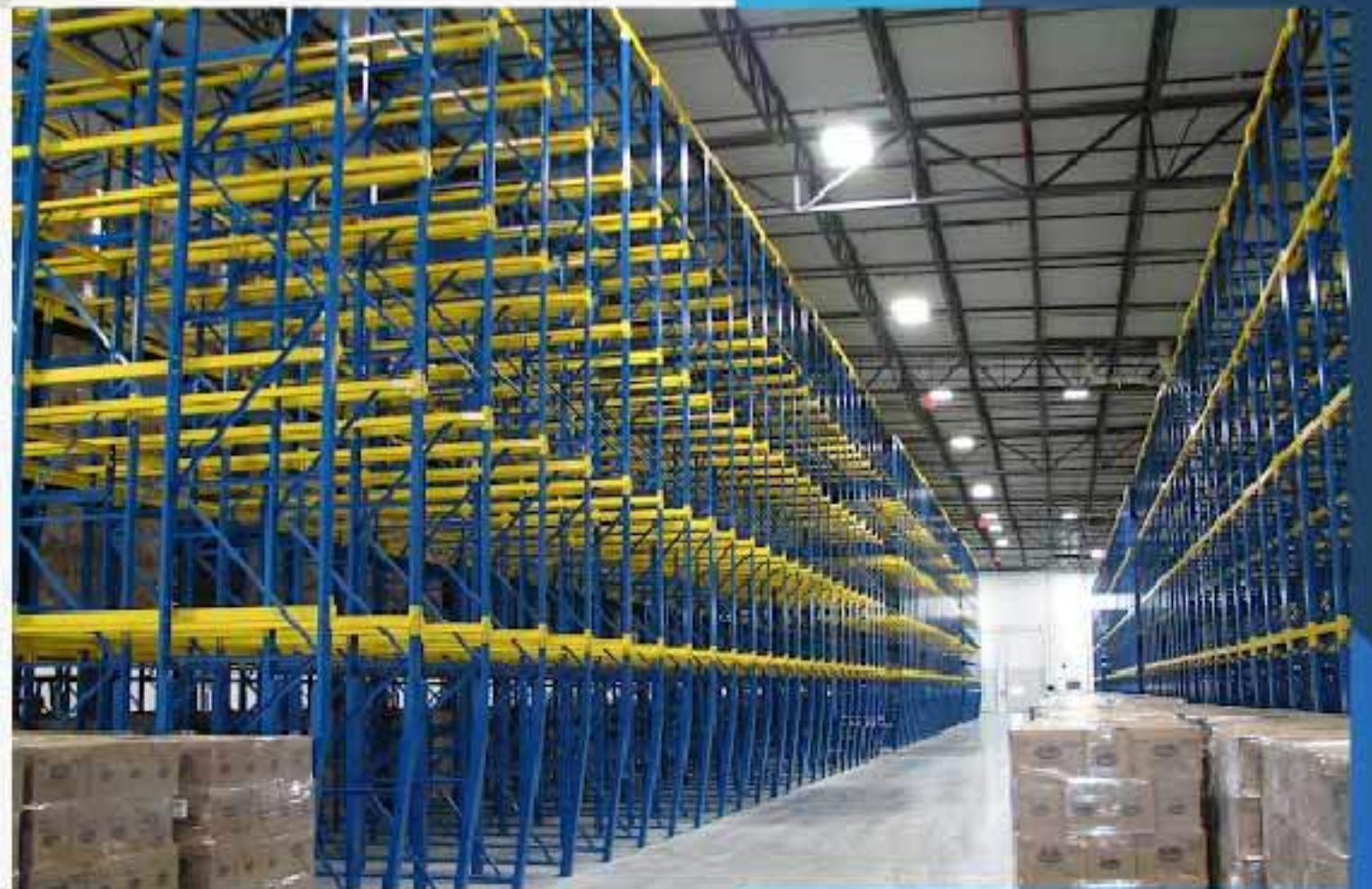
DRIVE-IN STORAGE RACK →
